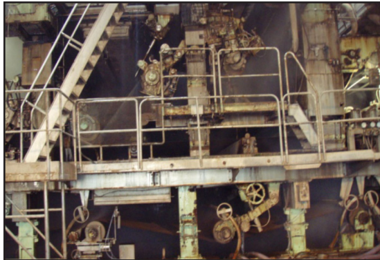
Corroded structure of old paper machine
